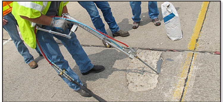
Cracks, spalls, static joints* and potholes are repaired instantly avoiding F.O.D. (Foreign Object Damage) *for dynamic joints use WVCO's EJC-25 expansion joint filler
